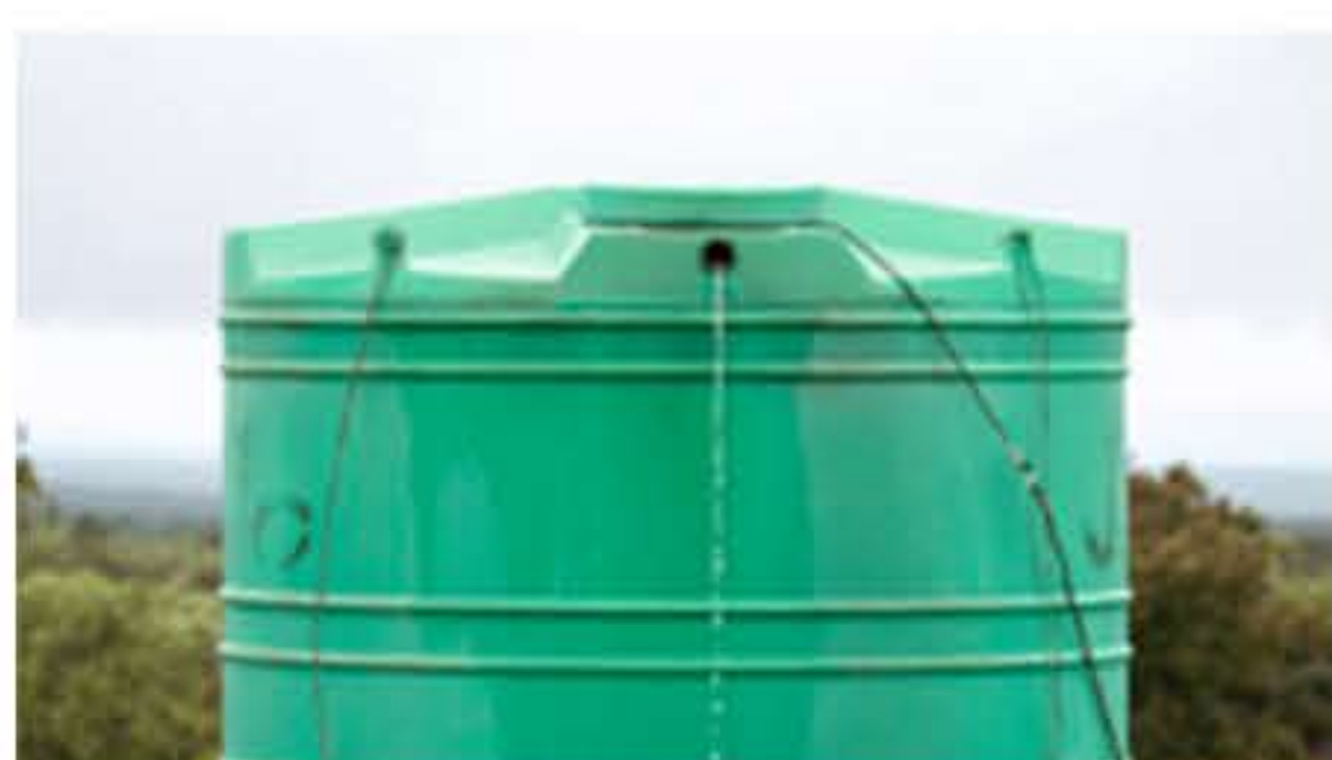
Tank level Monitoring
